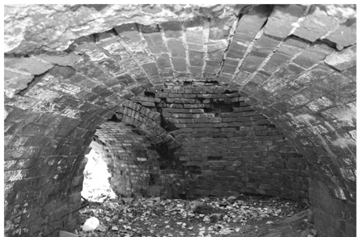
The base of the smoke stack for the Ashland Steel and Iron blast furnace, located on Sanborn Avenue.
